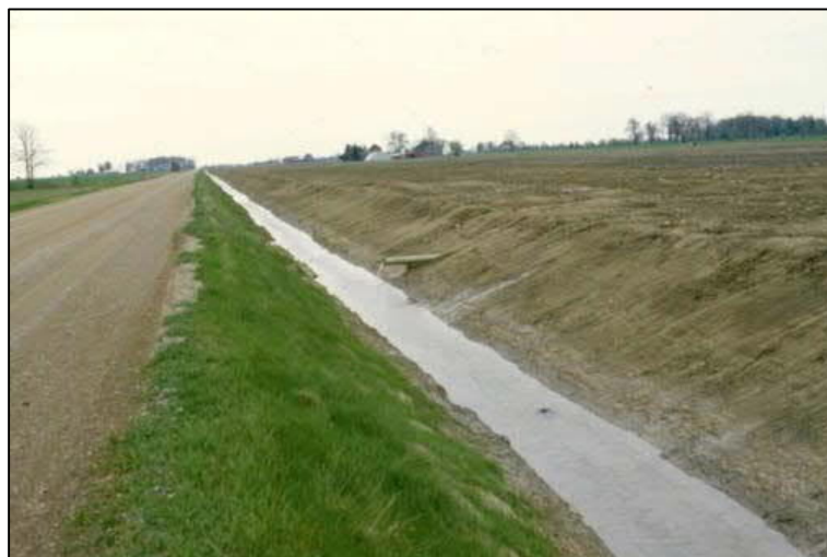
Figure 4 Example of clear drain
