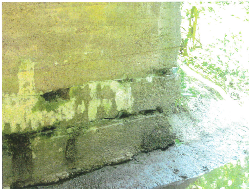
Large cracks on the north end of the west abutment wall
