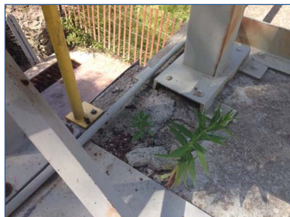
Figure 3: Localized Concrete Spall
