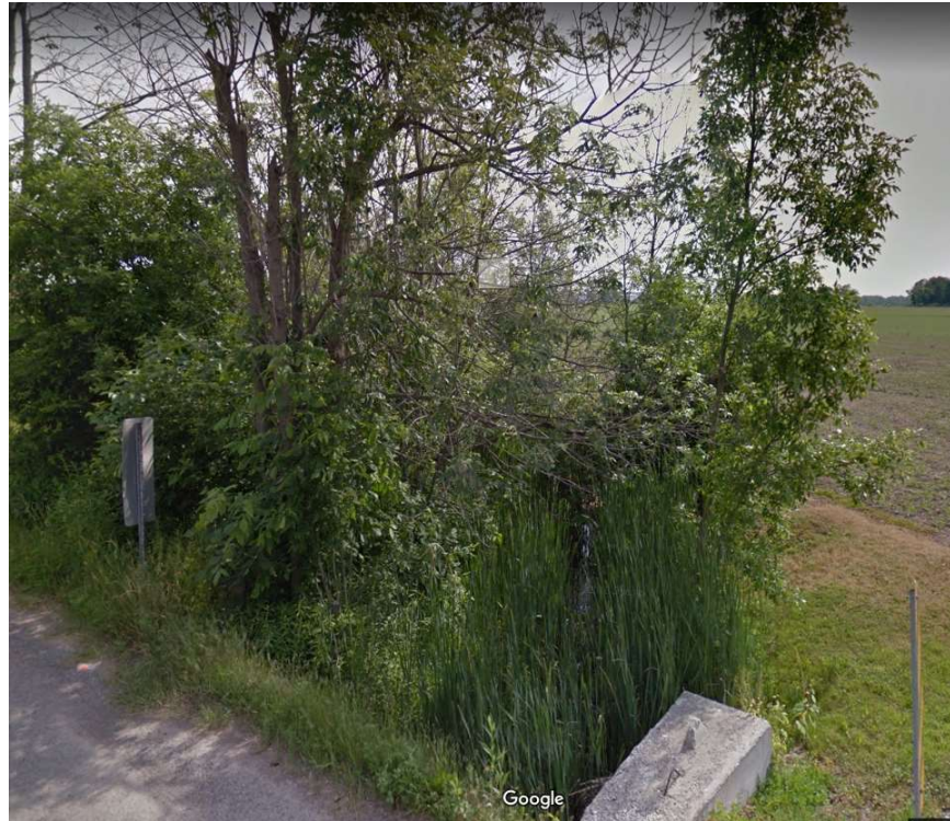
Figure 6 Vegetation obstructed drain
