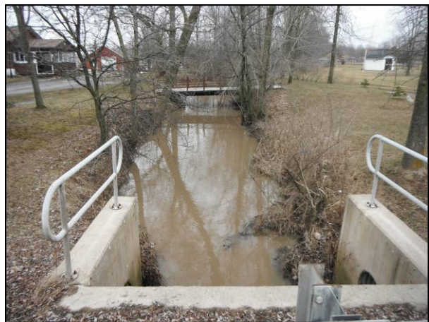
Photo 48: Reach 6a-B, Hwy # 3 culvert crossing headwall & lateral drainage (piped roadside ditching)pipinginterface. Former Geo. A. Schooley Award Drain. 16
