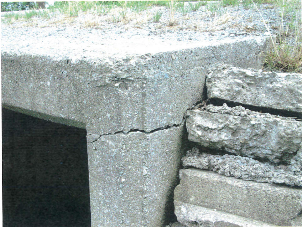
Cracking at the southwest corner of the structure
