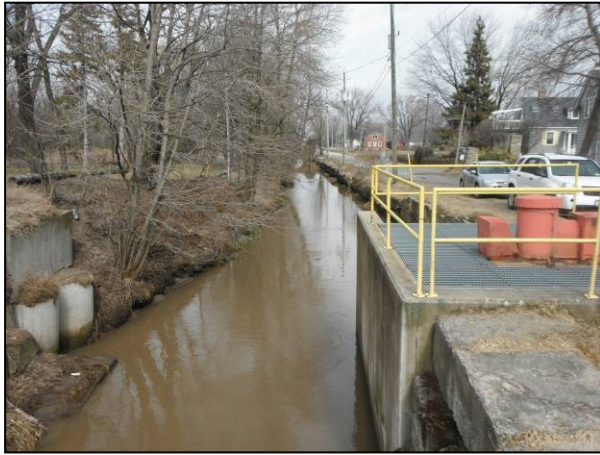
Photo 37: Reach 1-B, water control structure
