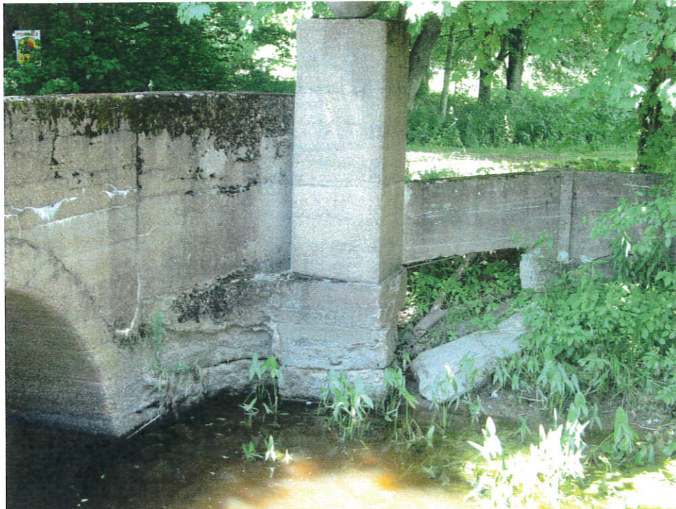
Concrete has deteriorated and broken away, at the northwest wing wall
